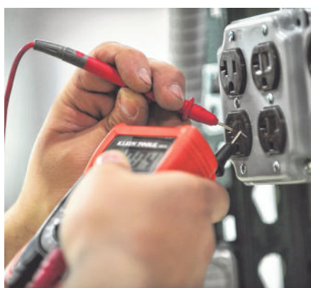
Top: Anthony Sanchez, 20, of Madison is an apprentice electrician for Esposito Electric. He uses a multimeter, above, to test that grounds are connected correctly and the voltage between the hot and neutral wires. KAREN MANCINELLI/CORRESPONDENT
