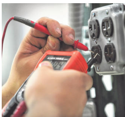
Top: Anthony Sanchez, 20, of Madison is an apprentice electrician for Esposito Electric. He uses a multimeter, above, to test that grounds are connected correctly and the voltage between the hot and neutral wires. KAREN MANCINELLI/CORRESPONDENT
